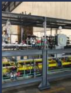
BOILER BURNER SKID
