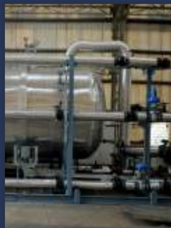
KNOCK OUT SKID
